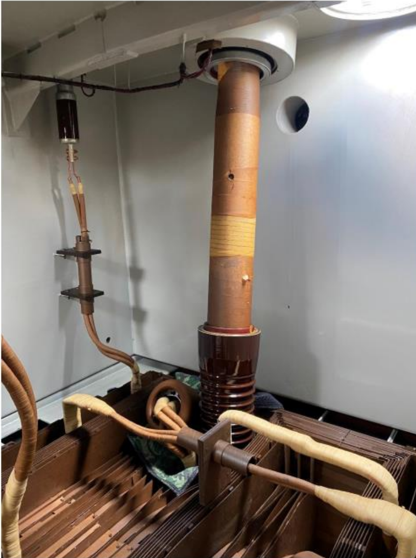
View inside tank of fallen lower bushing.
