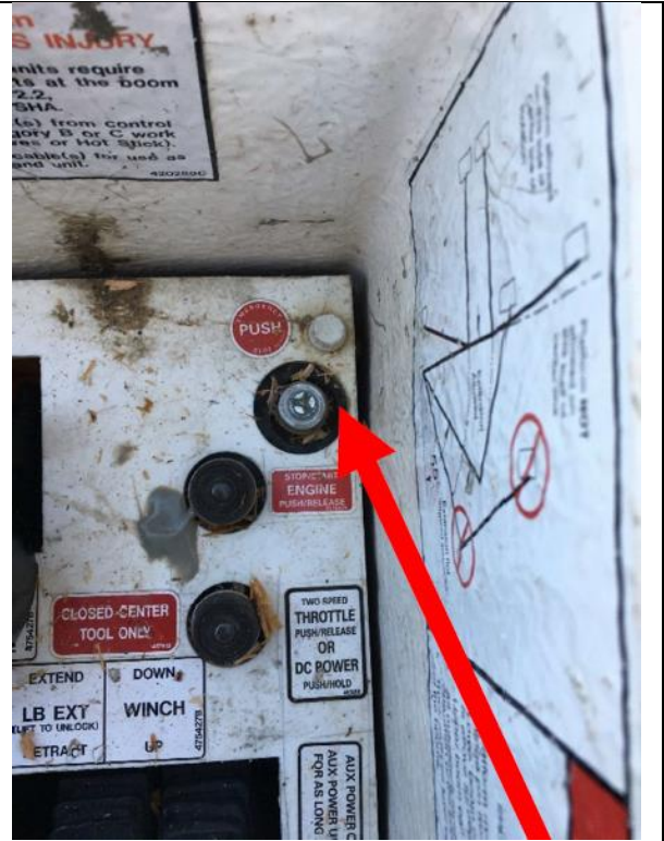
Bucket controls, with arrow pointing toward the emergency stop button.
